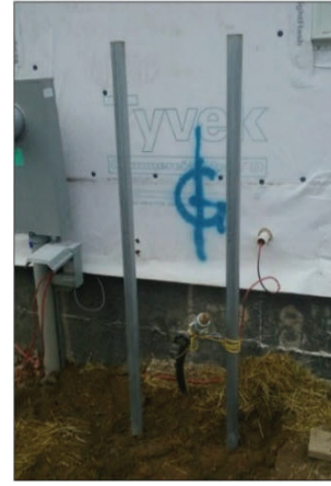
Freestanding/temporary meter post.
