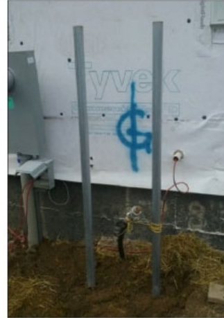
Freestanding/temporary meter post.
