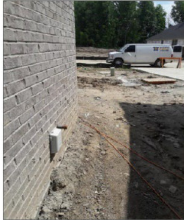
Clear pathway from meter location to gas main.
