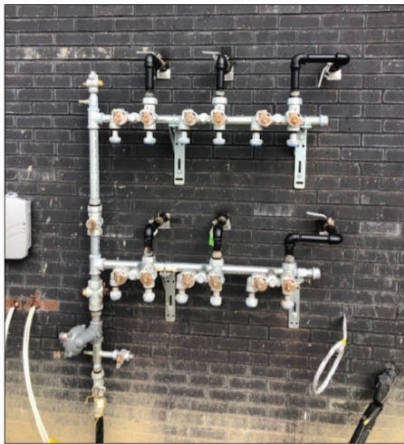
Multi-meter bracket showing Consumers Energy tags on fuel lines and service line connected to bracket.
