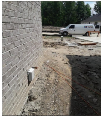
Clear pathway from meter location to gas main.
