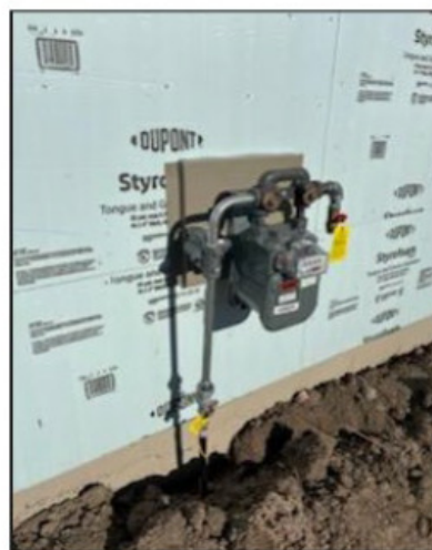
Meter mounted on a weather-proof permanent backer plate.
