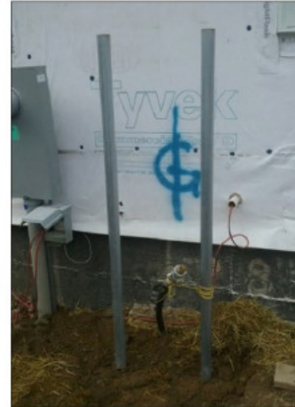
Freestanding/temporary meter post.
